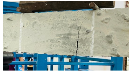
Figure 18. Crack On Beam
